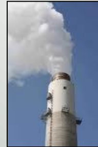
SCRs at Plant Miller 30 MW
